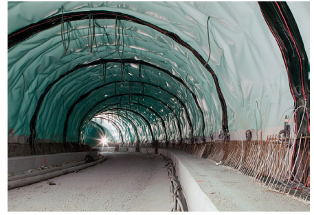
Fig. 26: Road tunnels present a very corrosive environment (de-icing salt and exhaust fumes from traffic).
