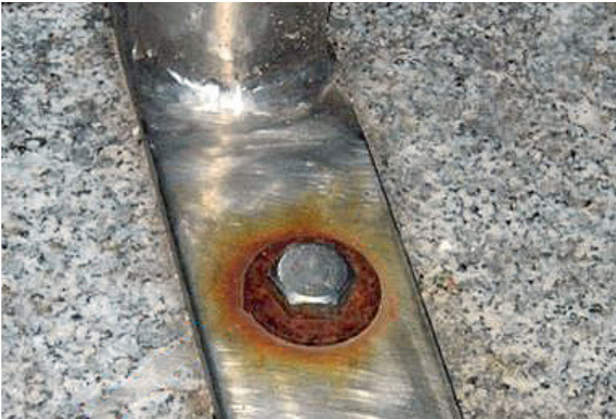
Fig. 12: This is a typical case of contact corrosion. A zinc-plated carbon steel (washer) and stainless steel (screw and part) were used together. The surface area of the more noble metal – the stainless steel – is larger, causing strong corrosion of the washer.
